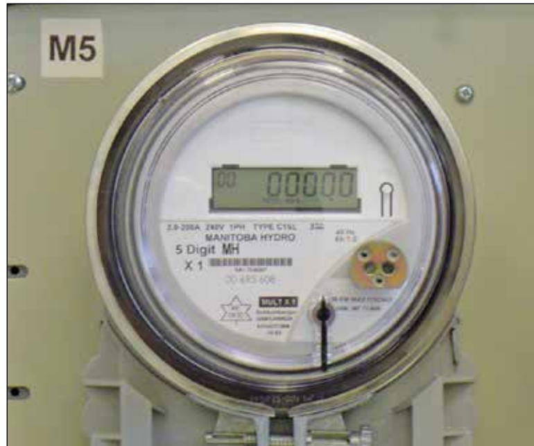
Pulse type load meter. This special meter monitored power consumption in the crates every 15 minutes, for an accurate picture of electrical demand and usage.
